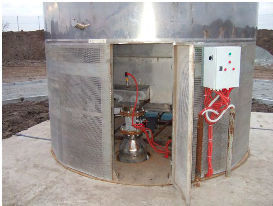
Enclosed ground flare (25 MW) with automatic ignition
