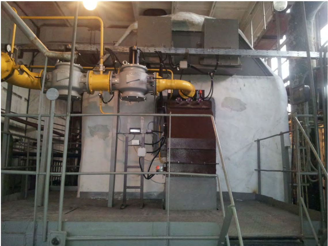
Steam boiler with MD Gas Burner of 30 MW capacity
