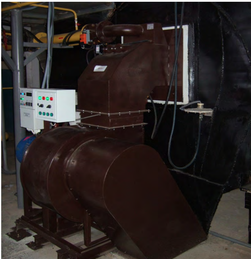
Steam boiler with MD Gas Burner of 12 MW capacity
