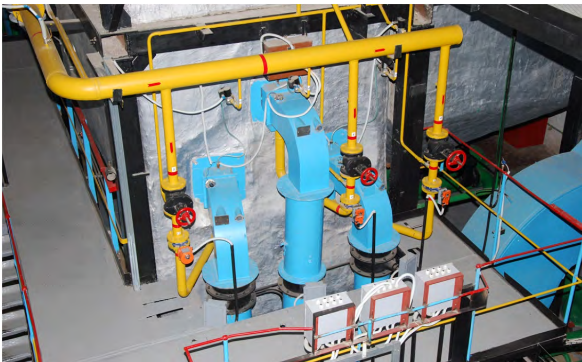
Steam boiler with MD Gas Burners
