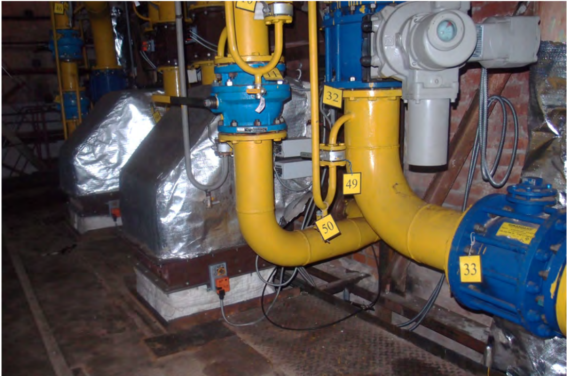
Steam boiler with MD Gas Burners of 20 MW (NG+Biogas)
