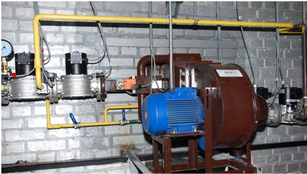
Heating Furnace with MD Dual Gas Burner of 3.0 MW capacity
