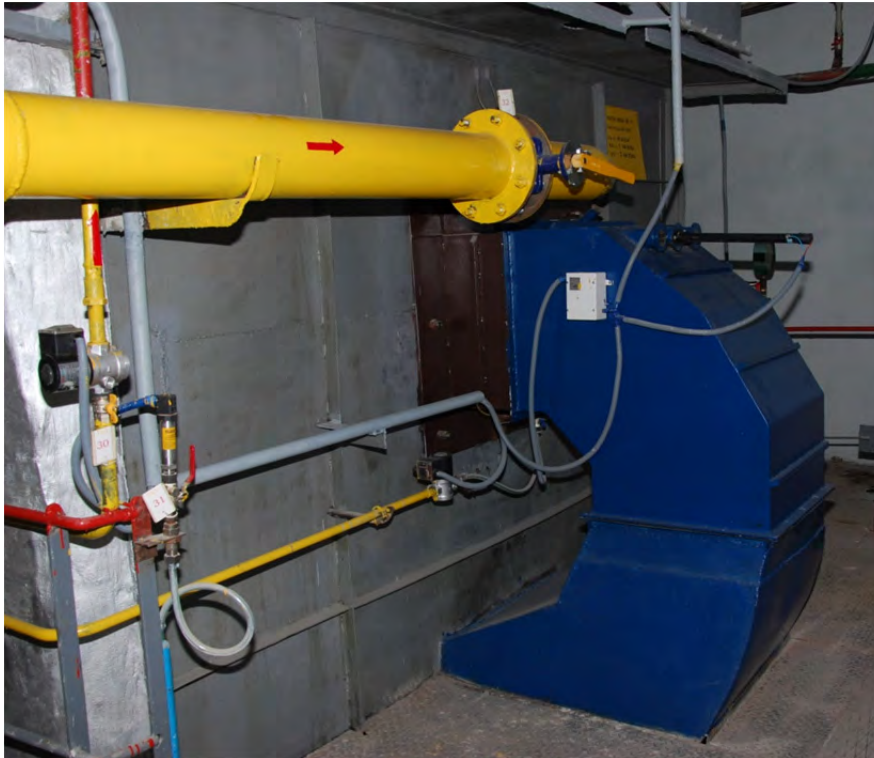
Water-heater with MD Gas Burner of 20 MW capacity
