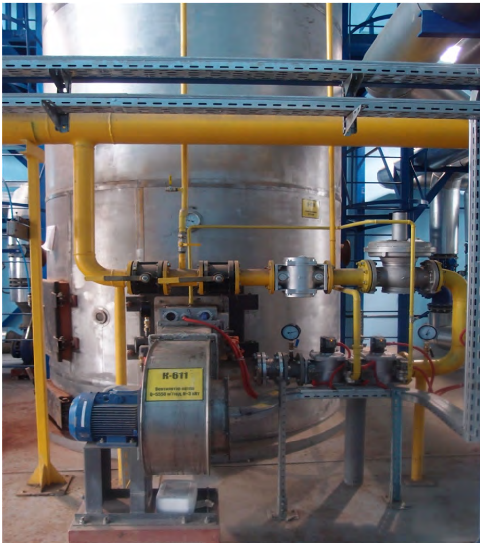
Steam boiler with MD Bio Gas Burner of 5.5 MW capacity
